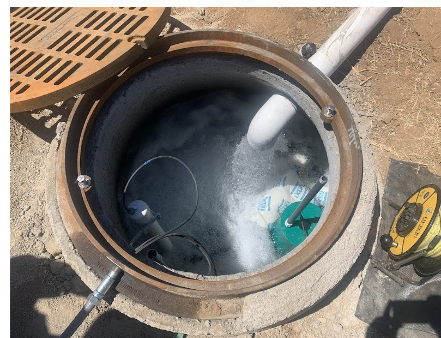
Recharge Well located in the Cosumnes Subbasin
