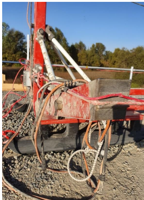
Figure A2-2 Close-up photo showing the transmitter frame mounted on the sled
